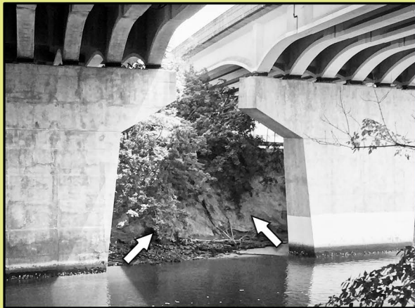
Extensive channel slope erosion
